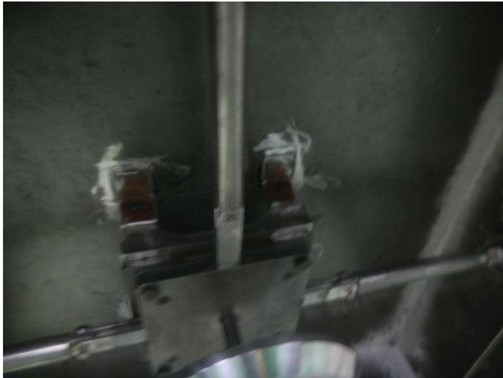
<PHOTO> WHETHER TO WATER LEAKAGE RESULT <ACCESS HOLE DOOR>
