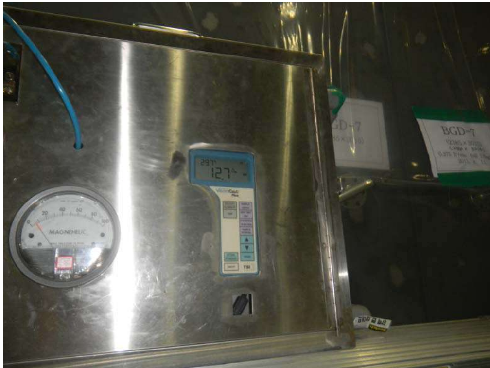
<photo> air leakage<BGD - 7>
